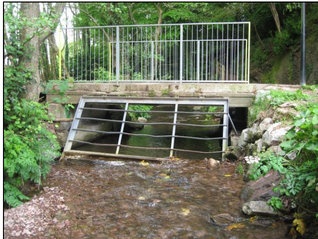
Plate 12: Ballybrack Stream showing bridge and trash screen in Ballybrack Woods, looking south
